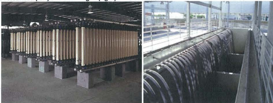
FIGURE 5-3 Pressurized (left) and Submerged (right) MF Installations
