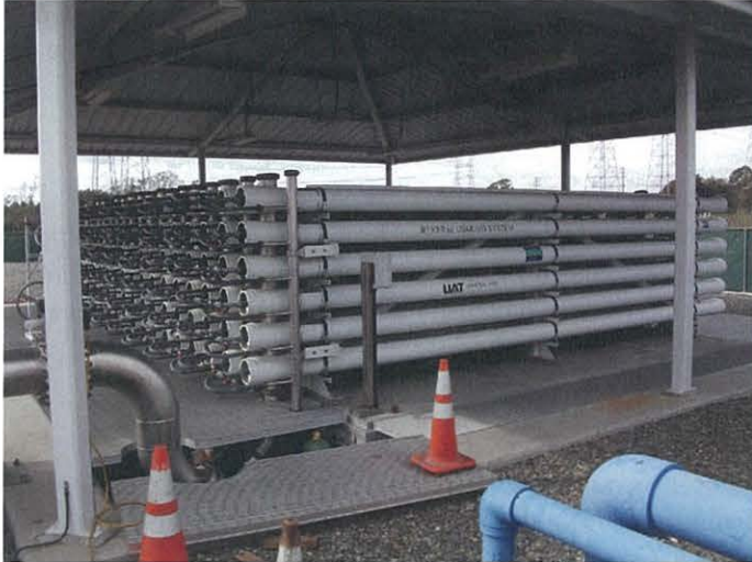
FIGURE 5-4 RO Pressure Vessels
